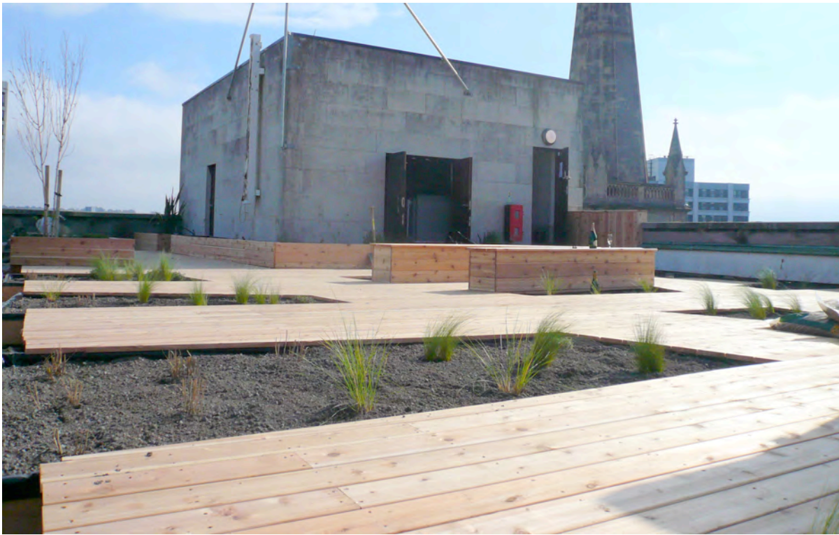
Shire Superlite substrate used as part of a vegetated roof garden in Bristol designed and built by sprout London & dmfk for The Office Group Ltd. picture by Nicole Gordon.
